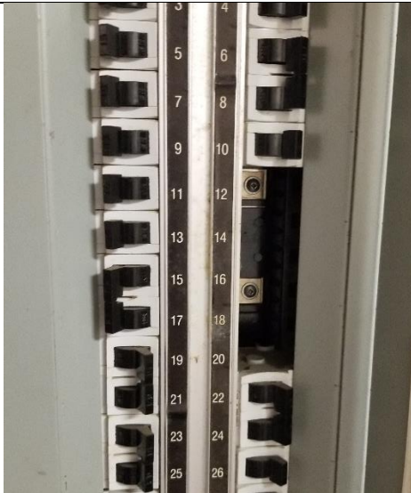
Figure 39 - Open electrical panel slots
