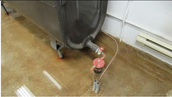
Figure 8 - Oil tank with bottom draw. Water ponding also noted.
