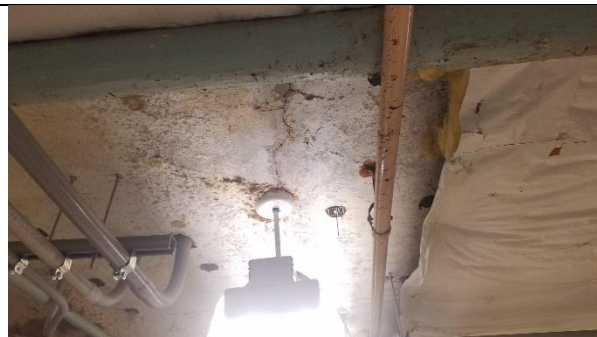
Figure 21 - Concrete cracks in the ceiling (main)
