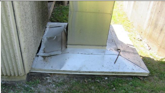
Figure 19 - Damaged external ducting
