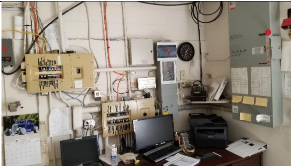
Figure 4 - Electrical panel obstructions
