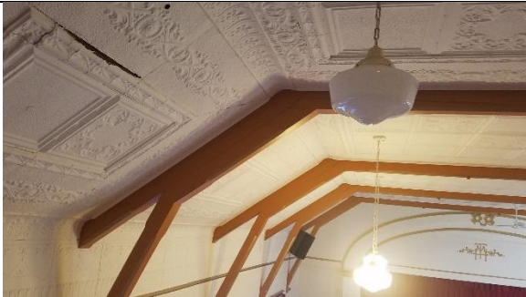
Figure 29 - Sign of Water ingress in the ceiling and indication of split in the aging structure
