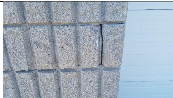
Figure 6 - Cracks in the joints of brick veneer
