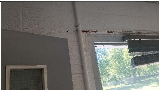
Figure 10 - Cracked and corroded lintel
