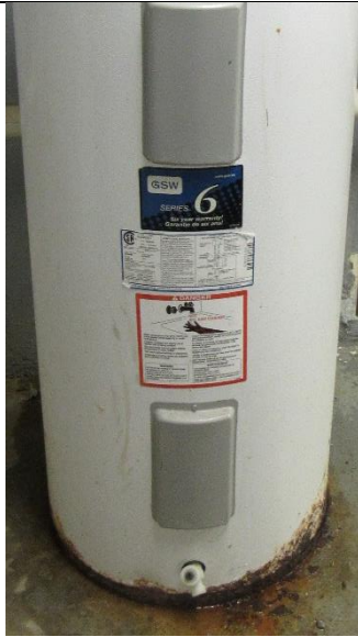
Figure 17 - Corrosion of HWT
