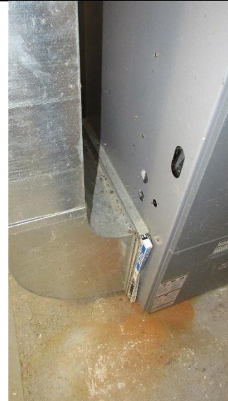
Figure 9 - Improperly sized furnace filter
