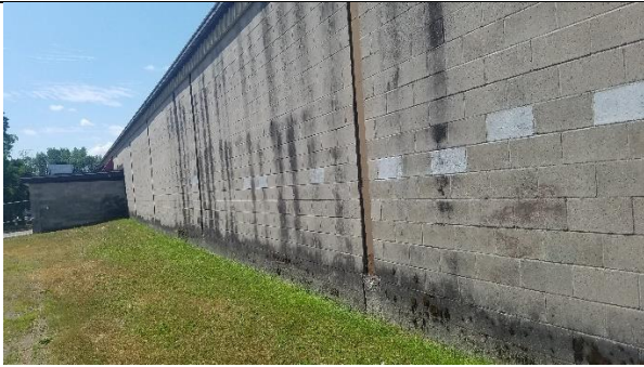
Figure 38 - Concrete elements deteriorated
