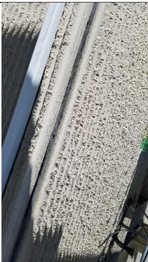
Figure 20 - Seal the joint of concrete panel deteriorated (main)
