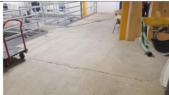
Figure 11 - Crack in the concrete floor
