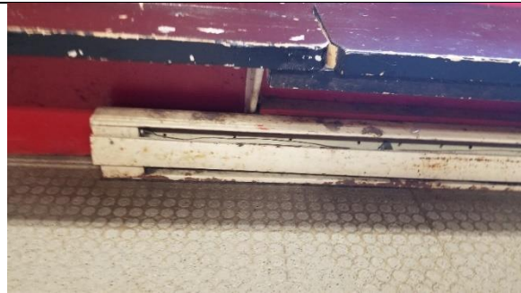
Figure 40 - Corroded baseboard heater
