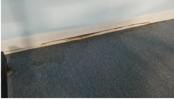
Figure 35 - Sign of water ingress in basement
