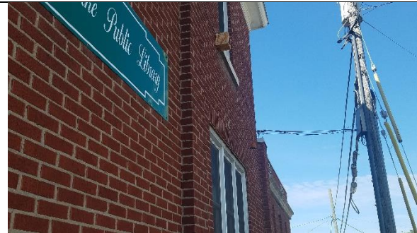
Figure 34 - Unused fixtures to be removed
