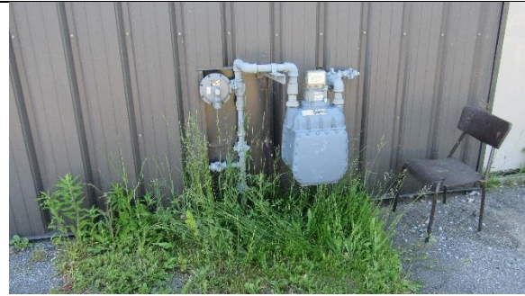
Figure 3 - Unprotected gas service
