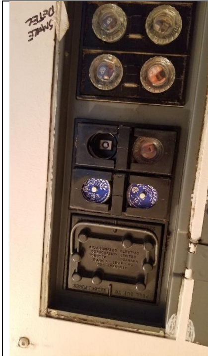
Figure 31 - Fuse panel for replacement
